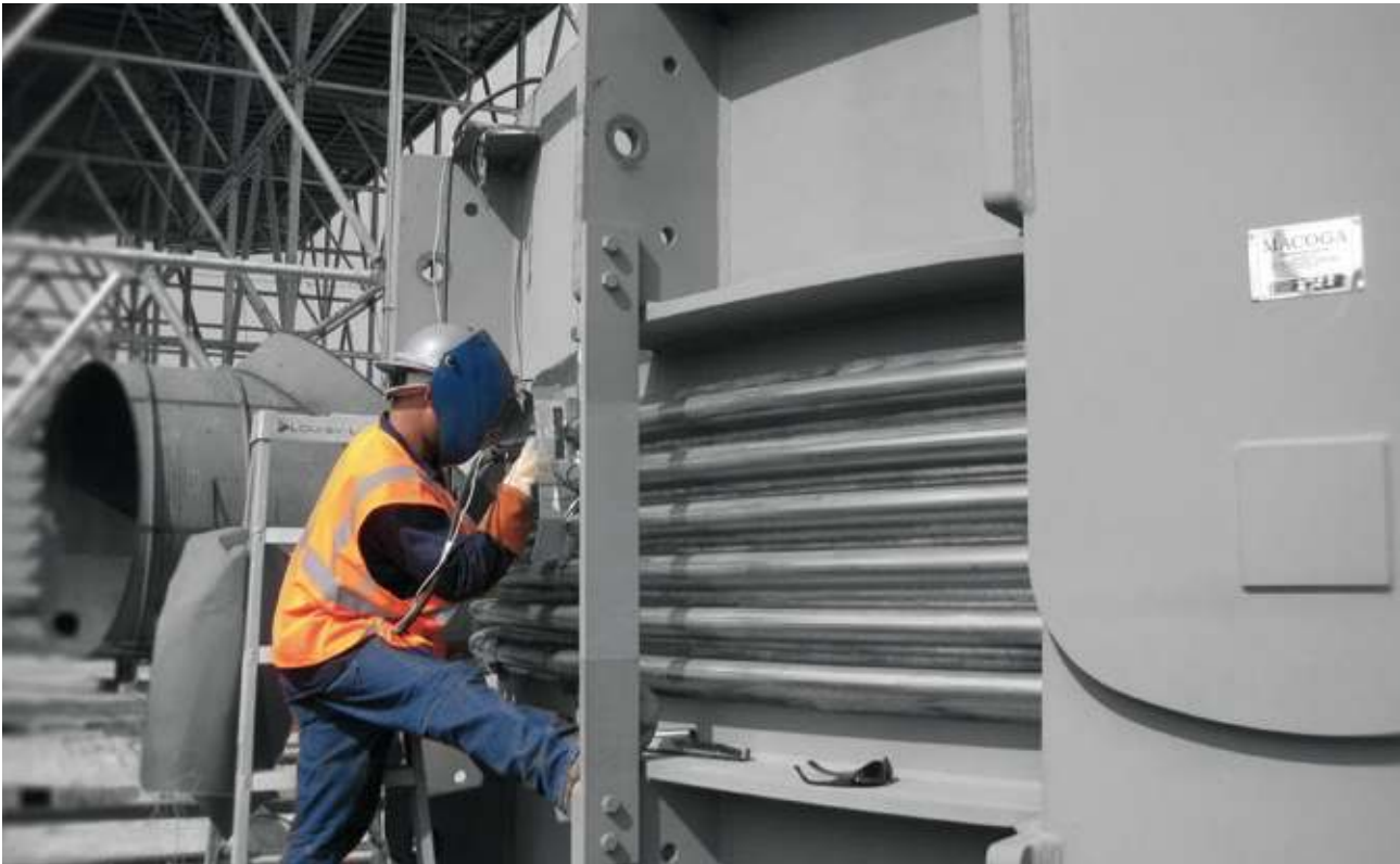
Assembly of a 7200 mm diameter MUX Expansion Joints in a Power Plant in Turkey
