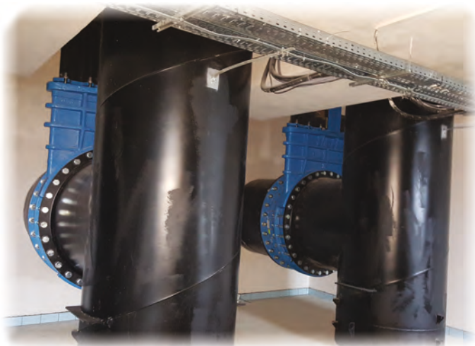
Clean water treatment application
