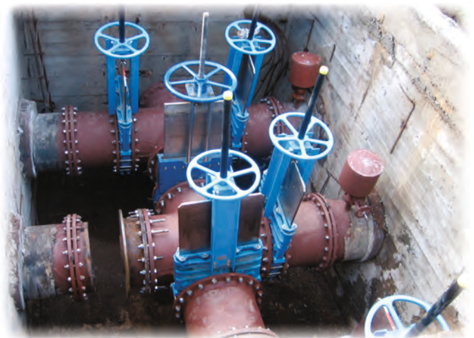
Sewage water treatment application
